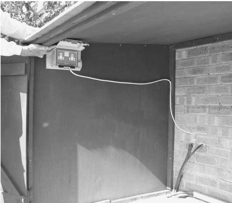
Figure 9.11. Electrical supply in the shelter.
