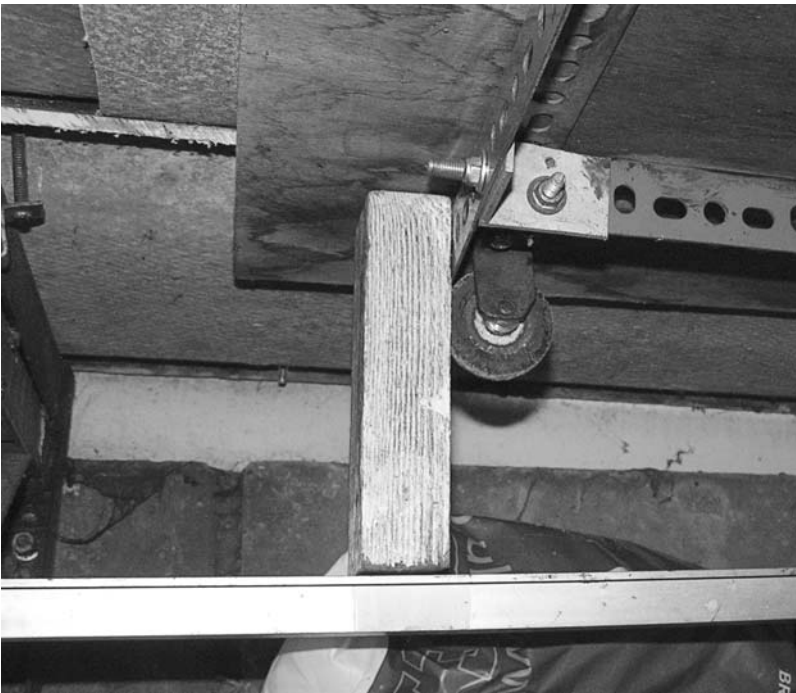
Figure 9.2. The rail and block arrangement holding up one corner of Bob's rolling roof, in the closed position.
