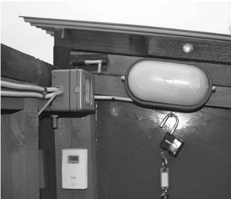
Figure 7.2. External sealed light fitting and switch.
