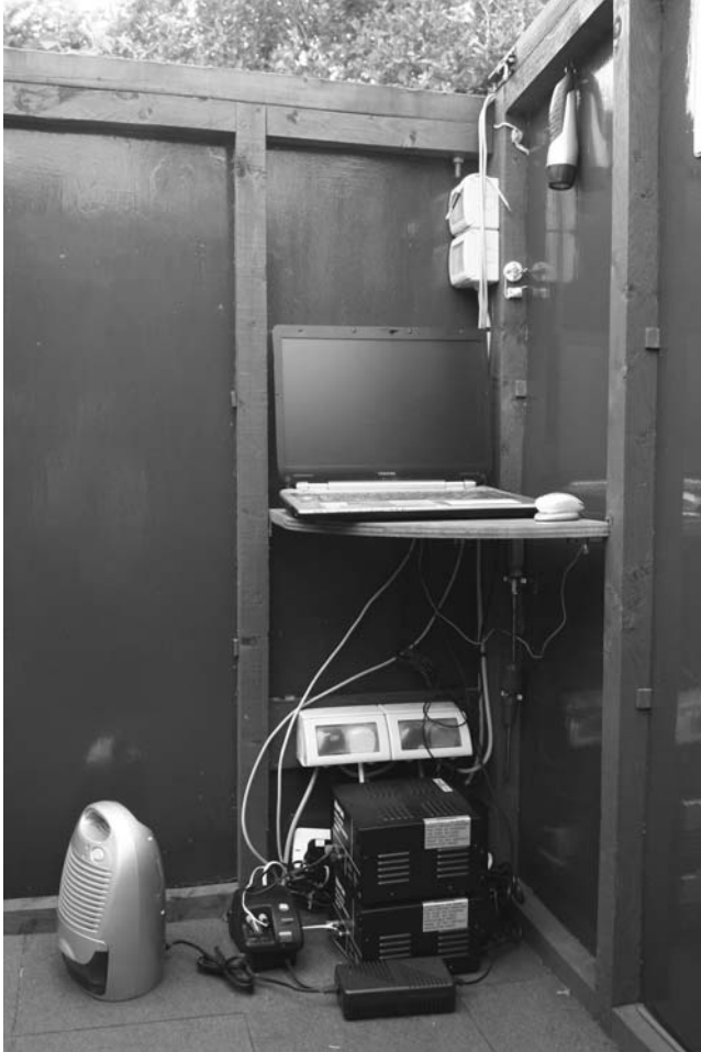
Figure 9.25. Computer shelf, power supplies, mains switches, and dehumidifier.
