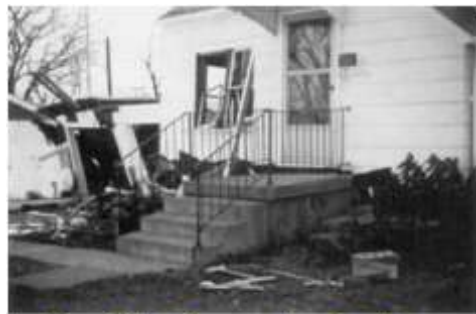
Low-Order Damage in a Dwelling.
